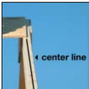
Be sure to attach plywood ridge boards at center line of rafter
