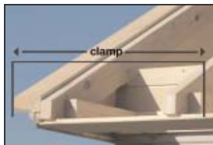
Use clamp at one end of the overhang to eliminate any gaps.
