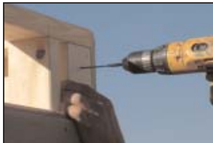
Screw the end panels through the attached 2x4s into the front and back panels.
